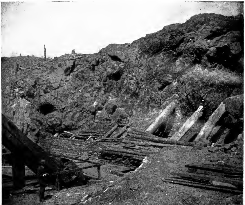
FIGS. 161 AND 162. —View of the Copper Cliff Mine, near Sudbury, Ontario. The mine is in diorite. The ridge at the background is granite. From photographs by T. G. White, 1894.
